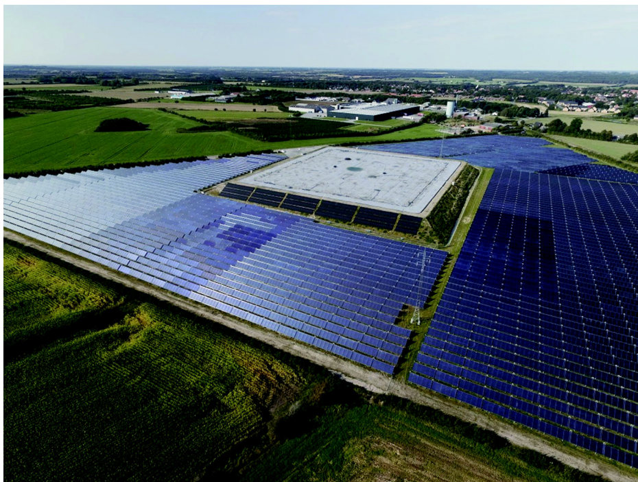
Figure 7 The solar water heating and heat storage pit at Gram district heating.
